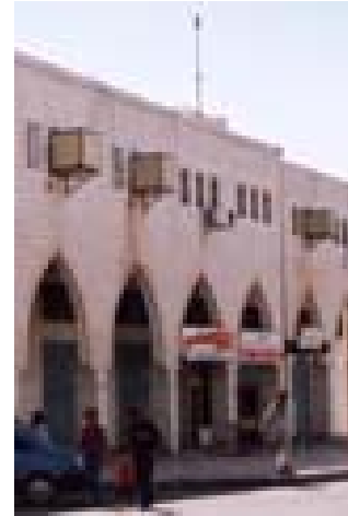
Photo (57) Air-Conditioning Split Unit - Jericho
